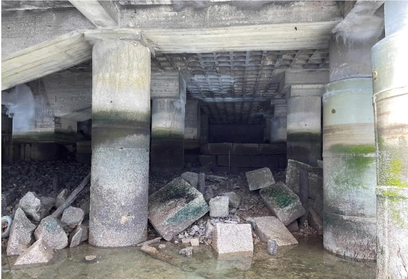
A – View of severely deteriorated granite seawall with rocky intertidal shores in front. Building concrete wall visible behind. Blocks are loose with large joints, many blocks are destabilized.
